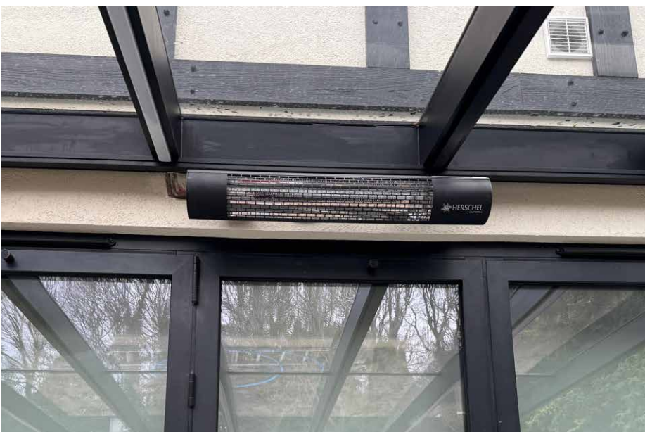
IMAGE SHOWING OUR CALIFORNIA HEATING SYSTEM IN POSITION ←
